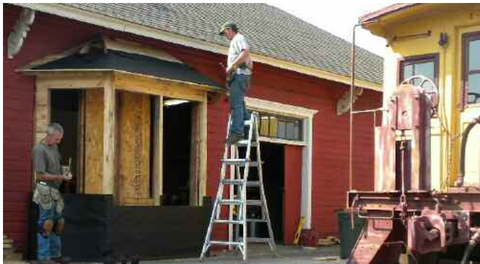
The Iola Depot station agent's bay window reconstruction was engineered by Charlie Wasrud (lower left) and installed with the assistance of his son, Ben Wasrud (on ladder), over this past summer.
